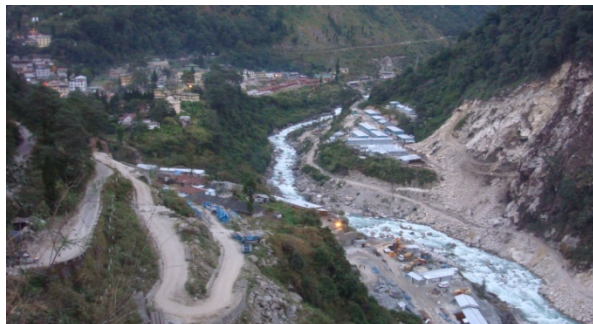
Power Project under construction at the Teesta River at Chungthang, North Sikkim
