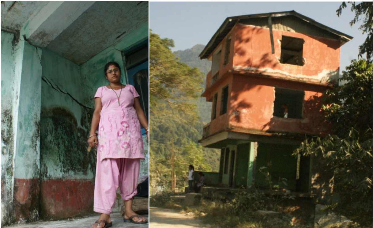
Almost 60% of the houses cracked, or many of them tilted at several locations all along the Teesta River due to tunnelling and also due to stop-and-go of dam water at Dkchu East Sikkim
