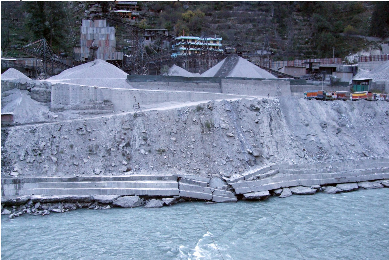
8. Photo showing the broken flood protection wall along the Sutlej River downstream of Karcham Wangtoo dam is broken leading to muck flowing into the river.. Photo taken on Nov 10 2010
