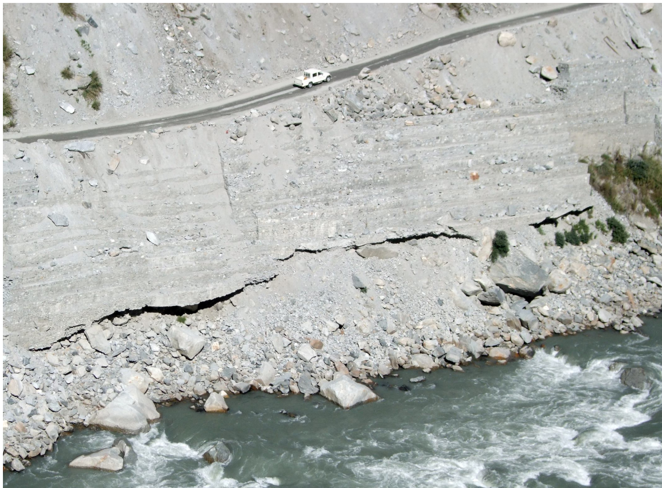
4. Photo 4 showing how the muck is flowing into the Sutlej river. Photo taken a few km downstream from the dam site on Nov 10 2010
