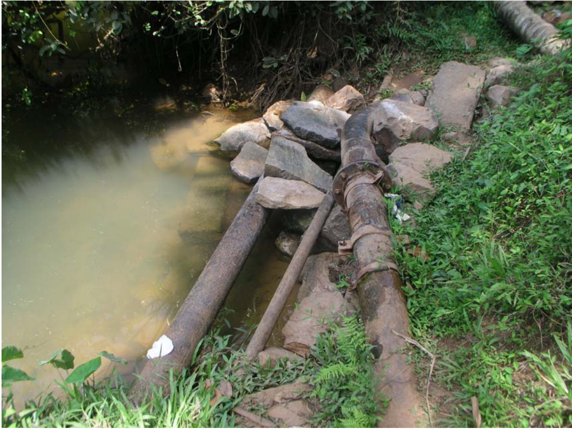
Leaky water distribution network: Source of contamination of treated water
