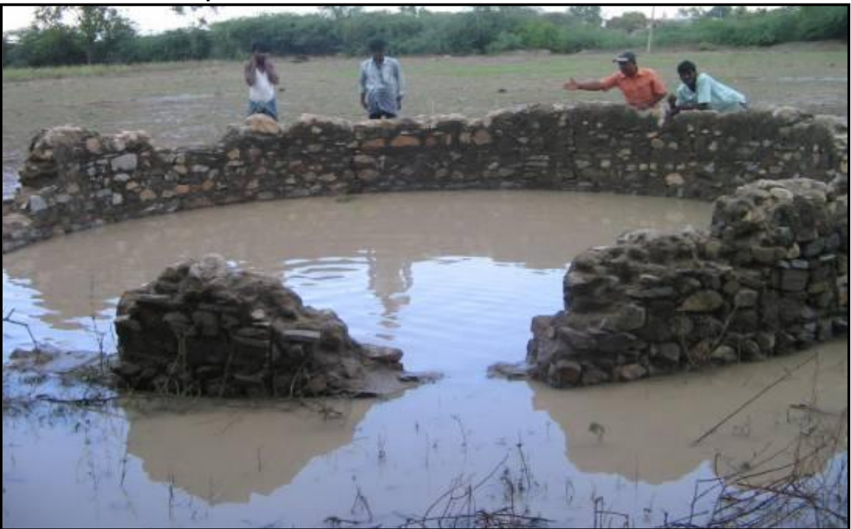
After intervention water from the well bottom was flowing like a fountain several inches thick that filled this dry well in 10 minutes
