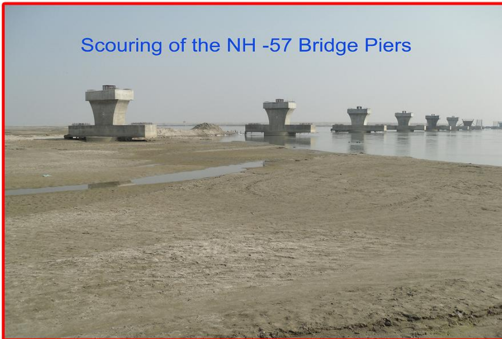
Photo 10. Scouring of the NH-57 Piers after the first Monsoon Floods in the River Kosi
