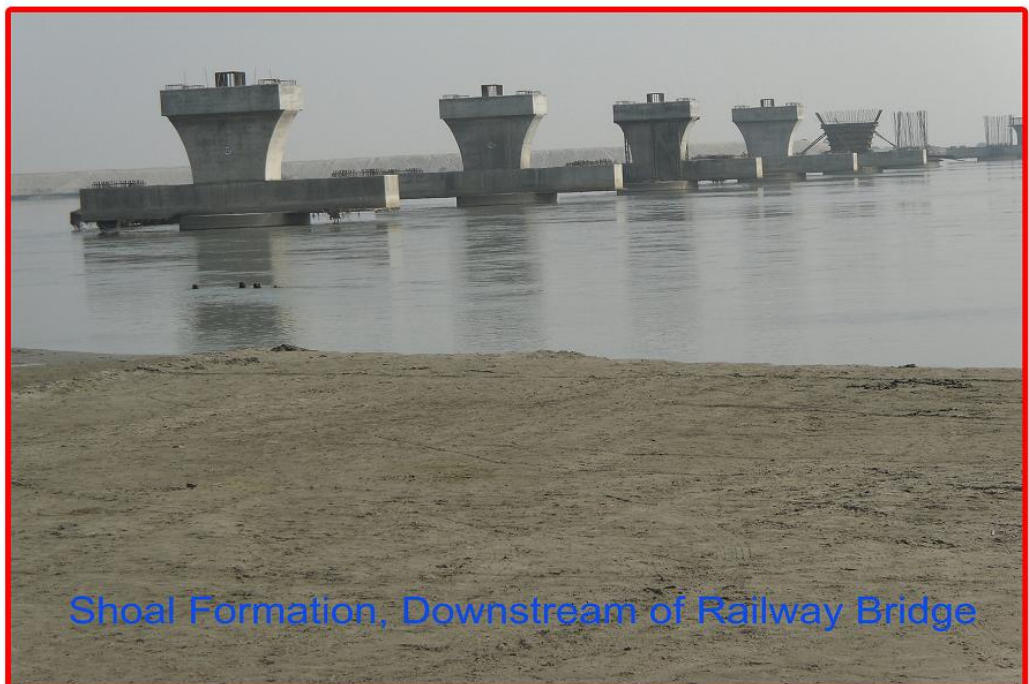
Photo 8. Shoal Formation Downstream of Railway Bridge Piers
