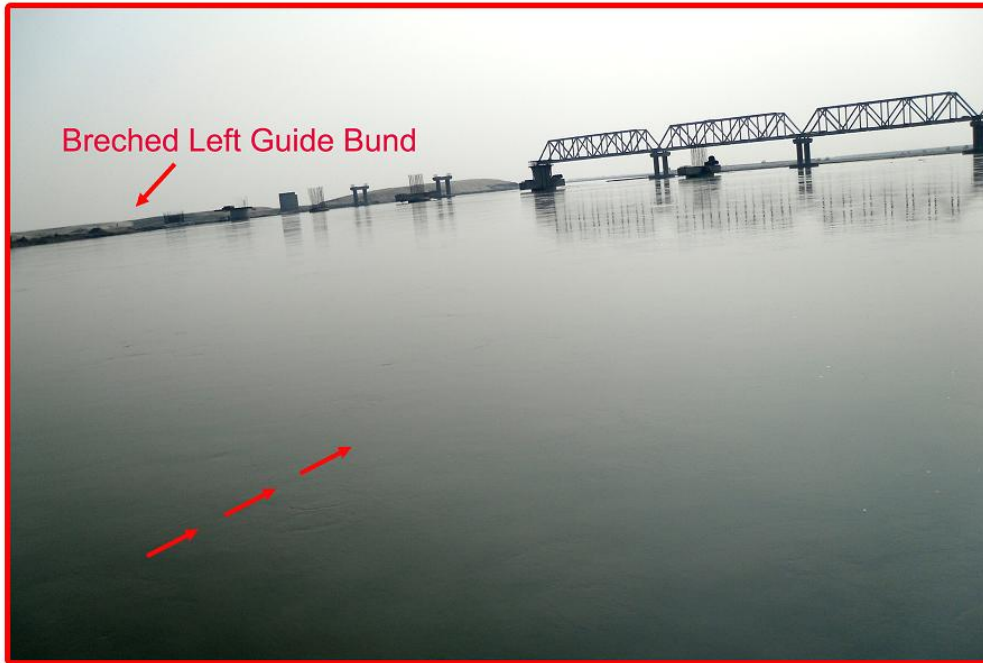
Photo 9. Breach in the Left Guide Bund
