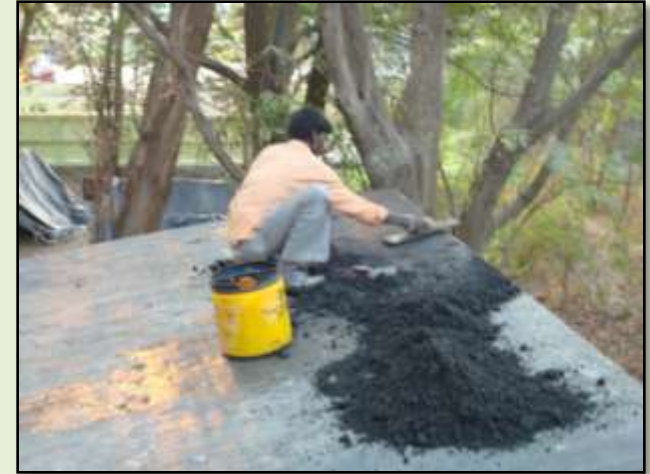
Application on the roof top
