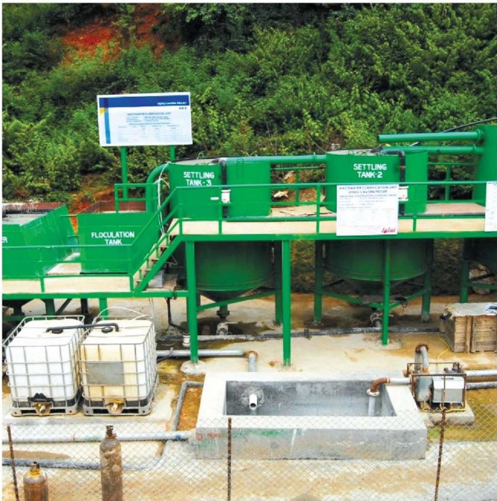
Wastewater Treatment Plant at Vizag Project site
