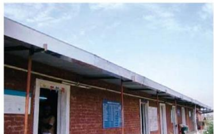
Rooftop Rainwater Harvesting at Mirzapur site
