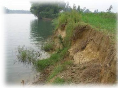
Figure 4-3: Bank before the vetiver implementation
