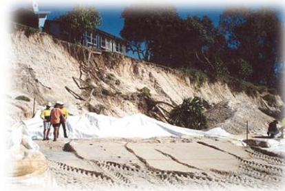
Figure 4-12: Bank before implementation of geo-bags
