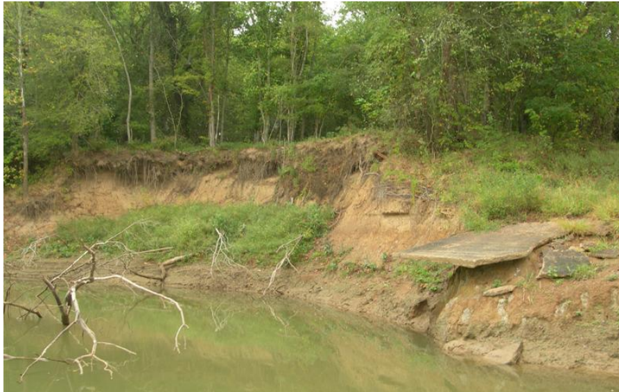
Figure 4-2: A typical eroded river bank
