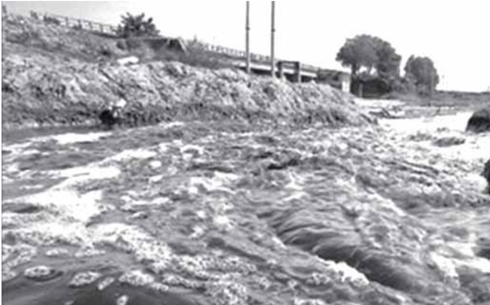
Figure 7 : Sea wall erosion
