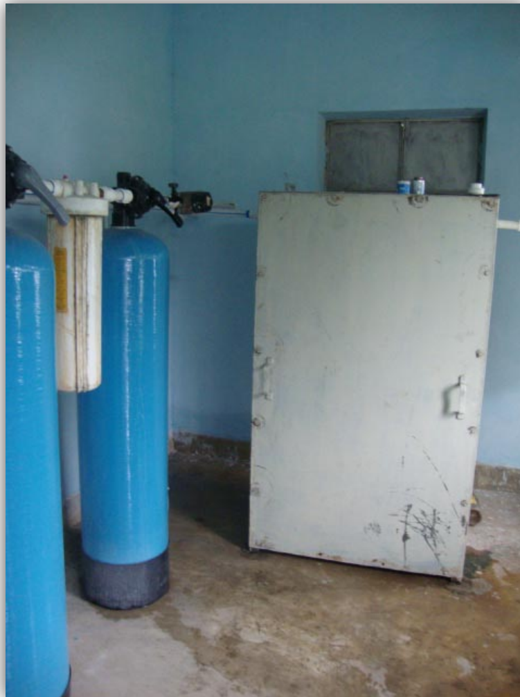
Figure 6-7: Interior of PHED solar based adsorption filter
