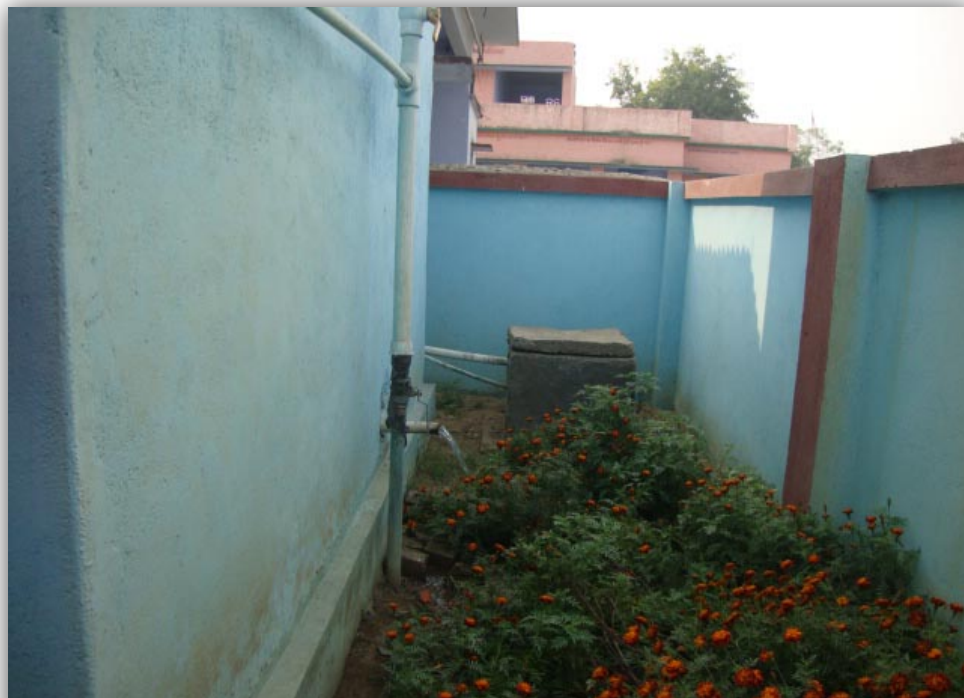
Figure 6-11: Sludge disposal of PHED Adsorption Filter
