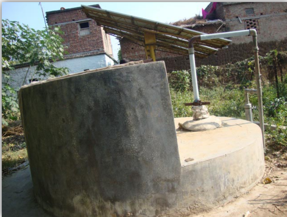
Figure 6-2: Solar based sanitary well
