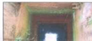
Banashankari Theertha, constructed in 1885, one of the big revived wells. Pic: Shree Padre.
