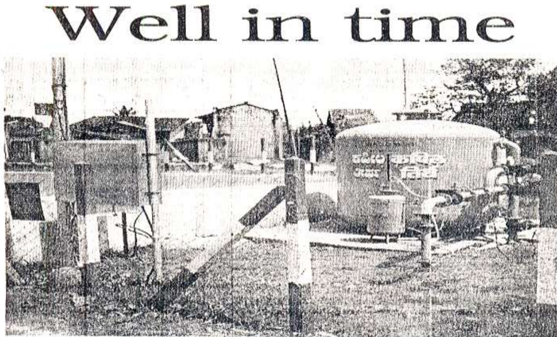
The filter unit at Kapila Theertha in Shahpur locality in Belgaum
