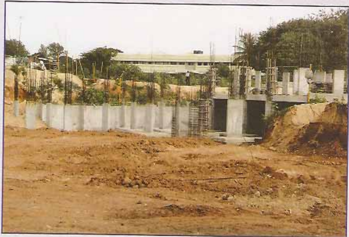
NIMHANS Land encroached by a builder
