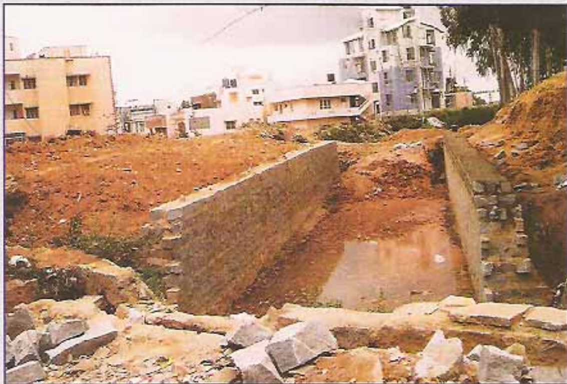
Encroachment of Raja Kaluve in Vibhuthi Pura, Bangalore East Taluk
