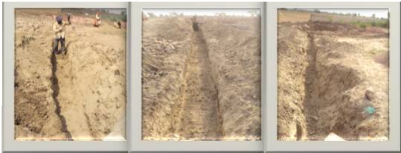
Underground drain (connecting drain inside the School Pond with that of the Cattle Pond)
