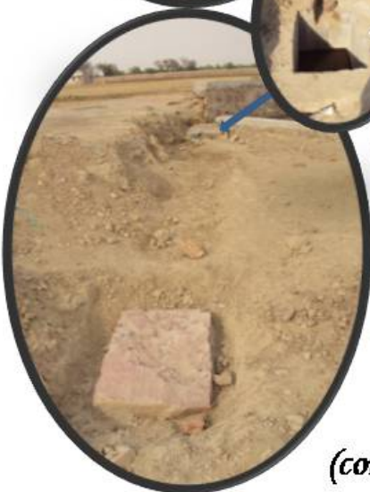
Chamber collecting drain water and passing it in the underground pipeline
