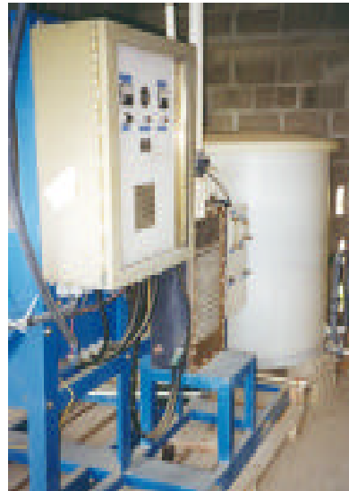
NaClO on-site production system for a 5,000 people community
