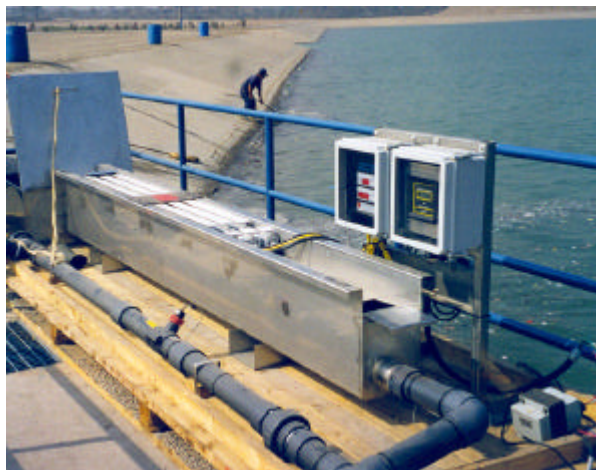
System using pipes parallel to the water flow in a drinking water treatment plant
