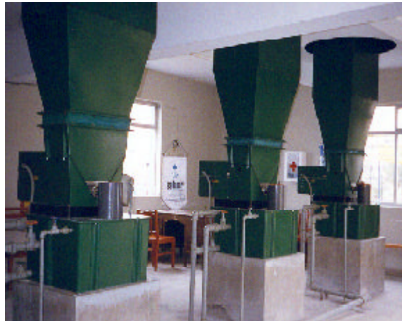
Dissolution feeders and tanks
