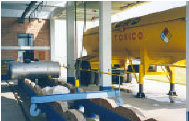
One ton cylinders and rolling tank containing chlorine
