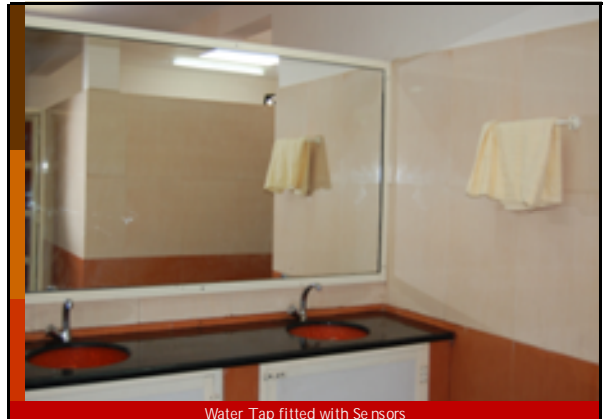
Water Tap fitted with Sensors
