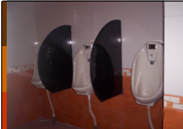
Urinals installed with sensor system, Bhopal, Madhya Pradesh
