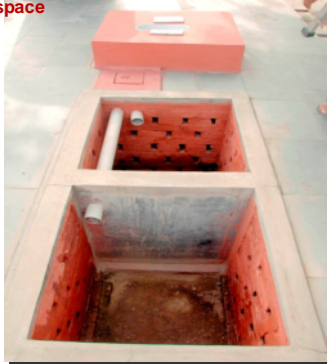
Sulabh pour-flush toilet for linear space with common dividing wall in a narrow lane 7
