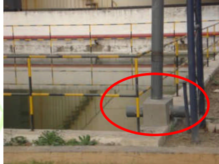
ROOF WATER STORAGE TANK
