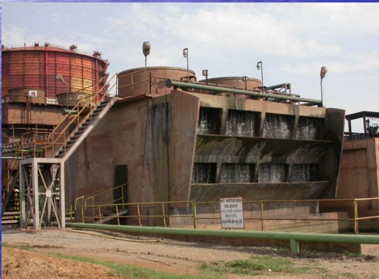
Higher COC in Cooling towers
