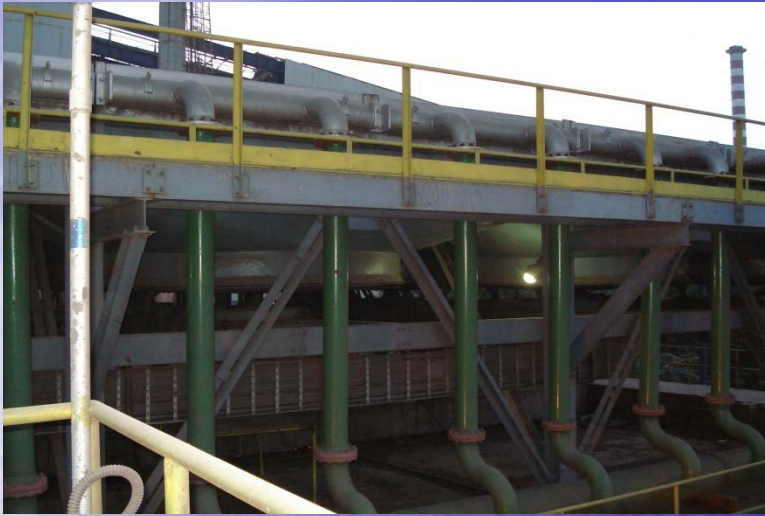
Fin-Fan heat exchanger
