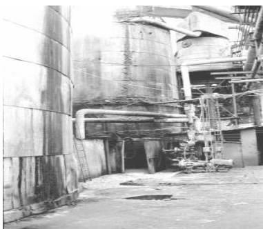
Figure 23.1. Leakages at a production plant
