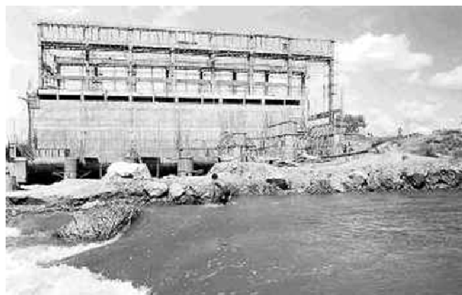
Figure 4.3: The unauthorised construction across the Tungabhadra near Sugur village (Source: www.bhinda.com 2004)
