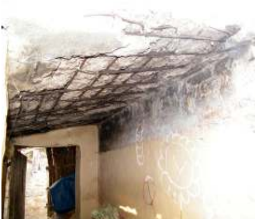
Fig 3.2 A degraded RCC ceiling. People neither have money nor the knowledge to maintain and repair these structures. Chatar Ghat, Khagaria District, Bihar
