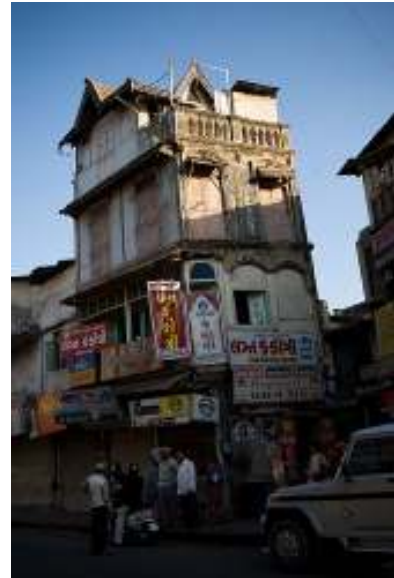
Figure3. 1: A leaning building. Recipe for disaster.
