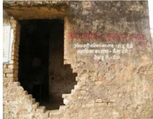
Fig 3.3 An Indira Awas Yojana structure which is degraded and falling apart being used as an Anganwadi.. Ilmas Village, Samasthipur District, Bihar
