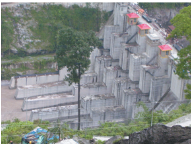
Construction of Teesta V Dam, Sikkim, India, 2008. India, with a huge planned capacity expansion of 50,000 MW in the next 10 years, will require funds to the tune of US$31 billion just in the next five years. Photo: River Basin Friends, India
