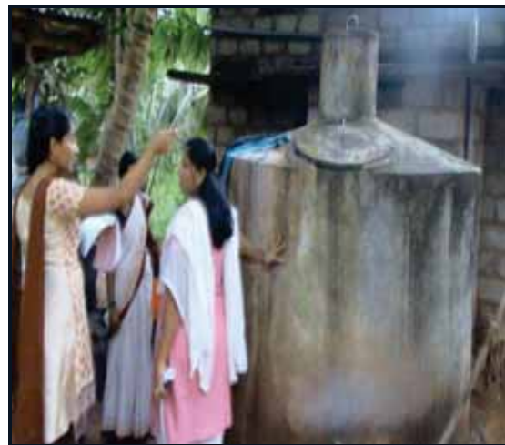
Rain Water Harvesting System in Punnamkulam
