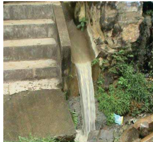
Over Flow of Water from the Pump House
