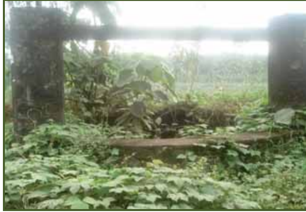
Poor Maintenance of Well
