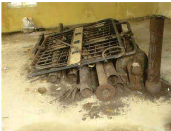
Improper Maintenance In The Pump House
