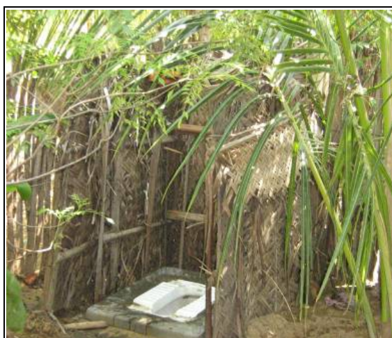
Toilet with temporary superstructure in Nainamaraikkan GP of Ramnathpuram in Tamil Nadu
