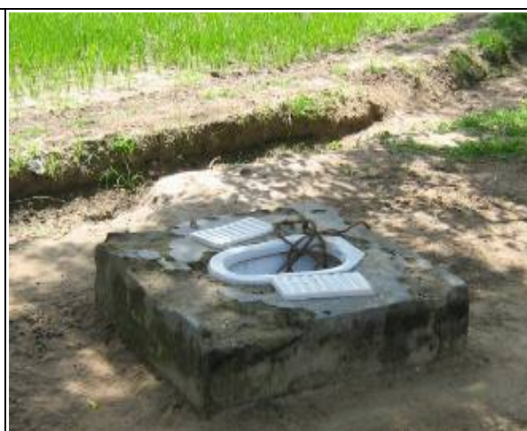
Toilet with no superstructure in Nainamaraikkan GP of Ramnathpuram in Tamil Nadu
