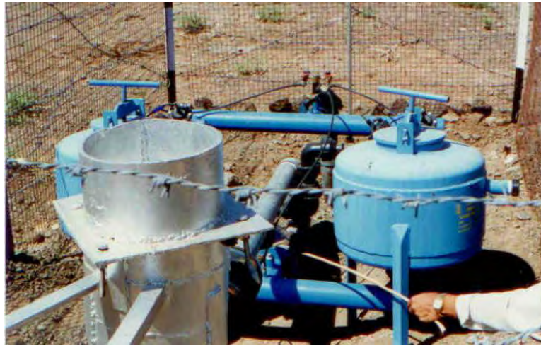
Figure.35 Injection well at Dambhurni, Watershed TE-17, Jalgaon District
