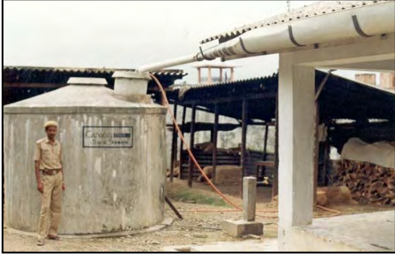
Fig-78 Rainwater harvesting tank in Portblair Jail
