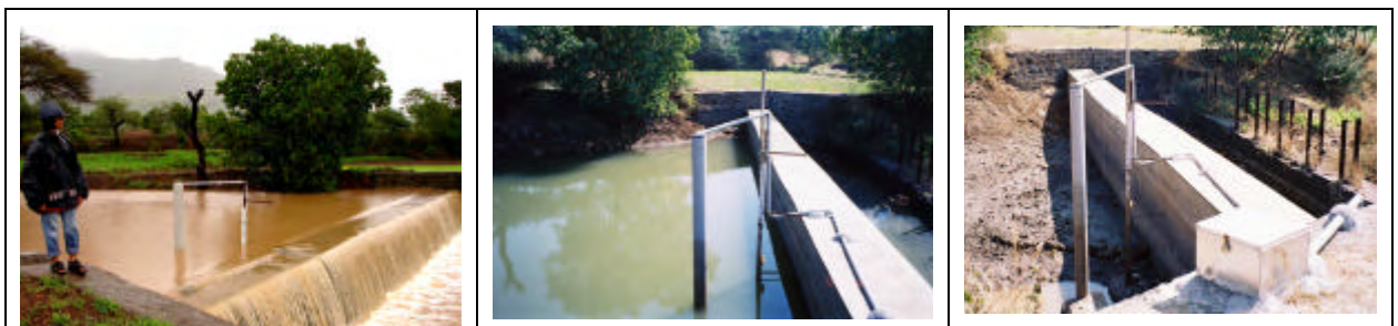
Check dam CD3 in different stages of monitoring shows overflow during the monsoon season (left), water level decline after the monsoon season (middle) and running dry in winter (right). The photographs show the monitoring set-up including a staff gauge and the stilling well with the data logger (in the box, right hand photograph).
