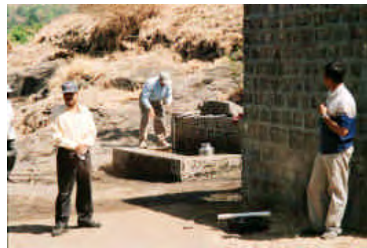
...feeds the water supply to hamlets downslope by gravity.
