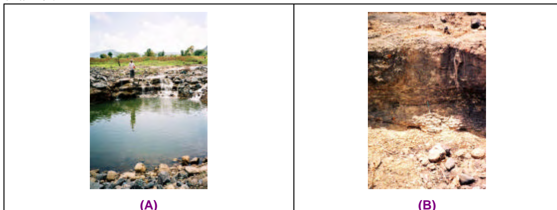
Dug well CH5, located on the Chikhalgaon watershed boundary is like a cistern (the basalt has limited permeability) and fills up very quickly with surface water (A). The same basalt unit, near the stream, is weathered and shows sheet joints (B).
