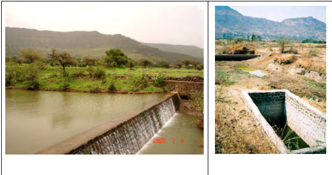
Check dam CD2 overflowing during the monsoon season (left) and drying up in early summer (right). The photograph on the right also shows dug well CH4.
