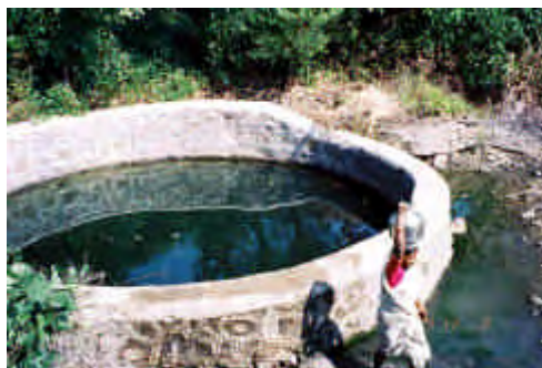
This well, in the Harijan vasti of Chikhalgaon, was repaired to provide drinking water to the hamlet that is about 500 m east of Chikhalgaon village.
