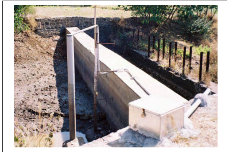
Staff gauge and automatic water level recorded (stilling well) in CD3, Chikhalgaon
