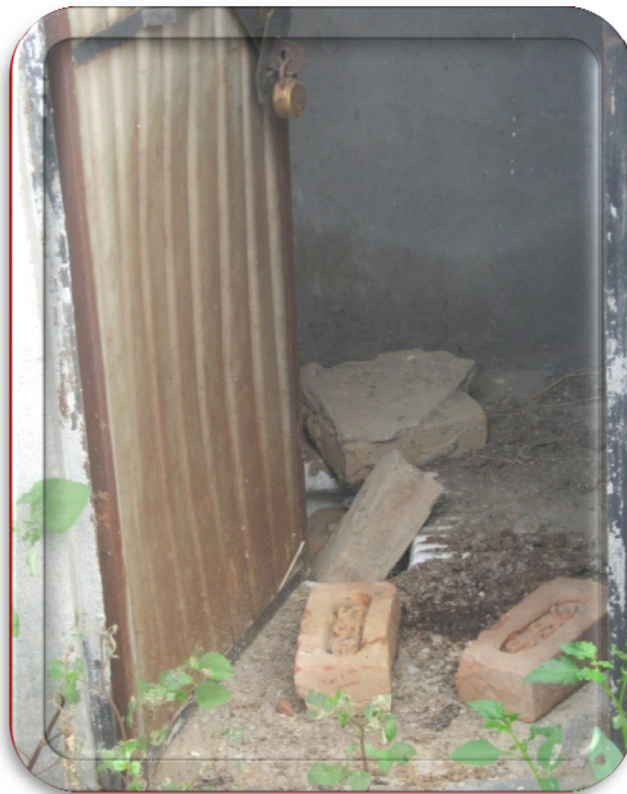
NON FUNCTIONAL TOILET FILLED WITH DEBRIS IN BIRMATHANA GP
