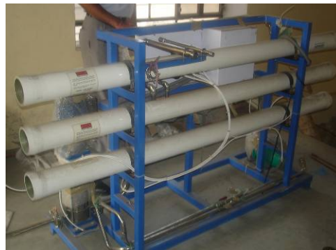
Water processing unit ( RO )
