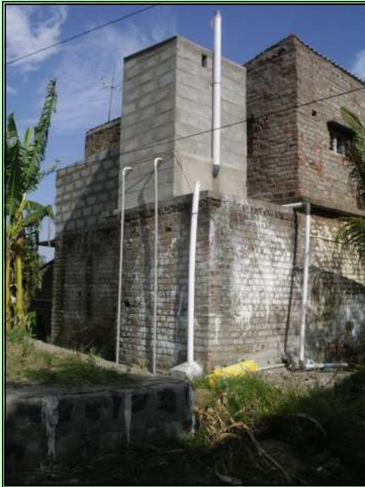
A view of the HCEST with separate pipe line for mud pot and filter bed.
