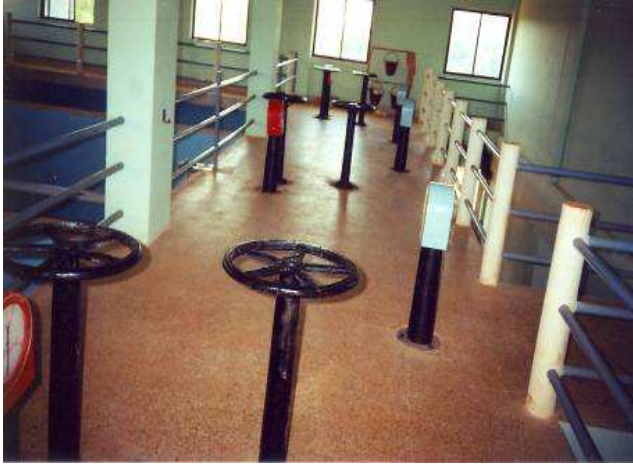
Filter House at WTP
