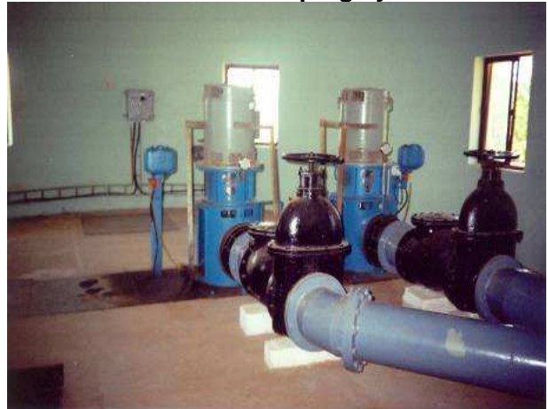
Raw water Pumping system
