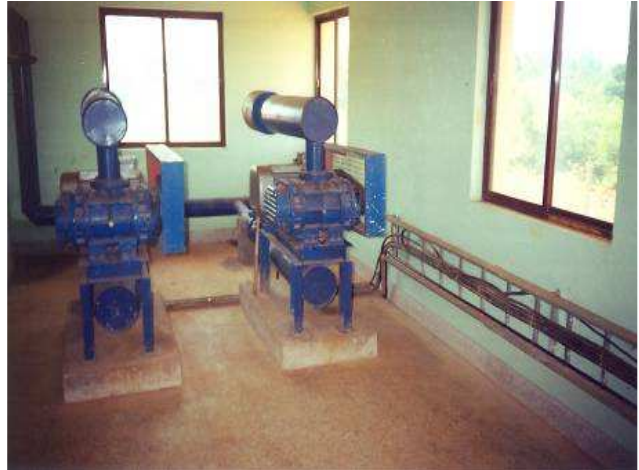
Blower of WTP
