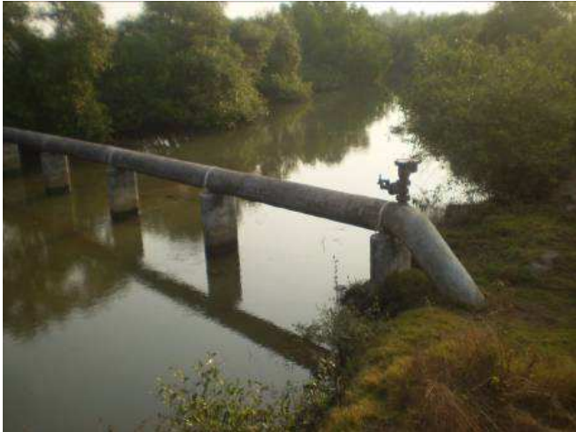
Clear water Transmission Main
