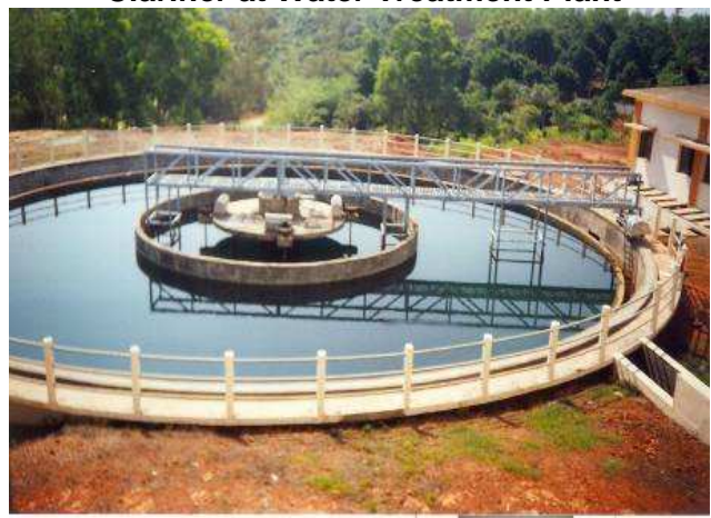
Clarifier at Water Treatment Plant
