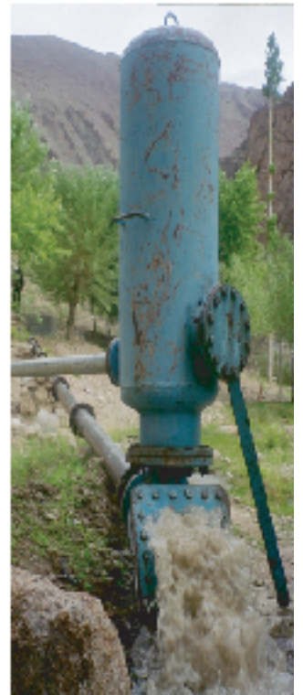
An installed Hydram in Ladakh
